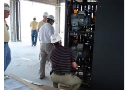
Checking the Liebert Unit
